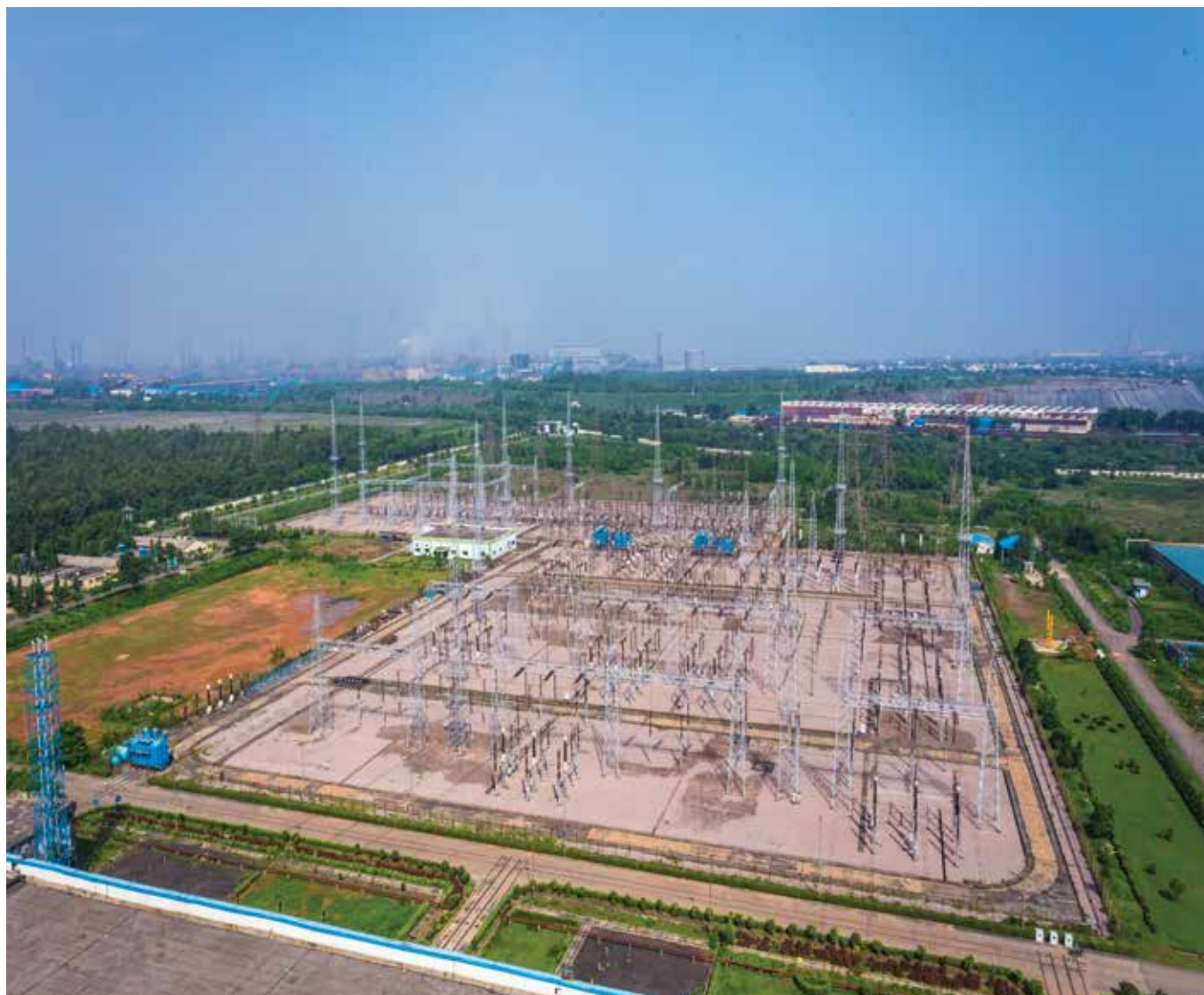
Switch yard Bhilai Expansion Project
