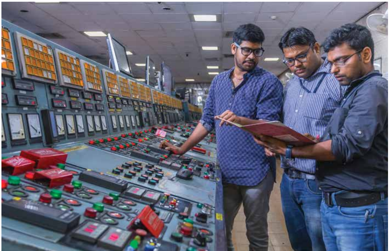
Control Room NSPCL Durgapur
