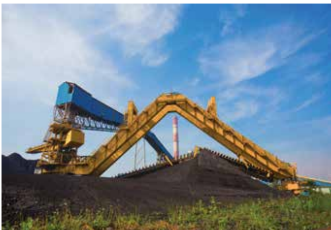
CHP Bhilai Expansion Project
