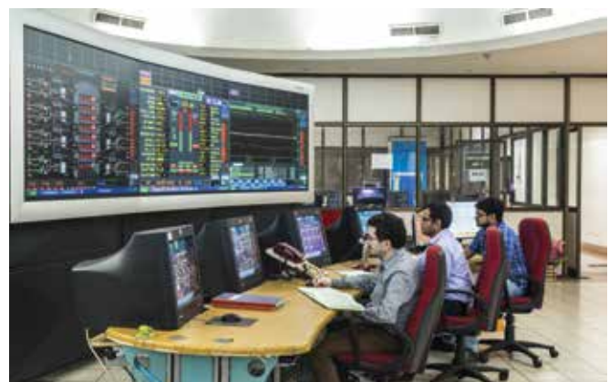
Control Room Bhilai Expansion Project
