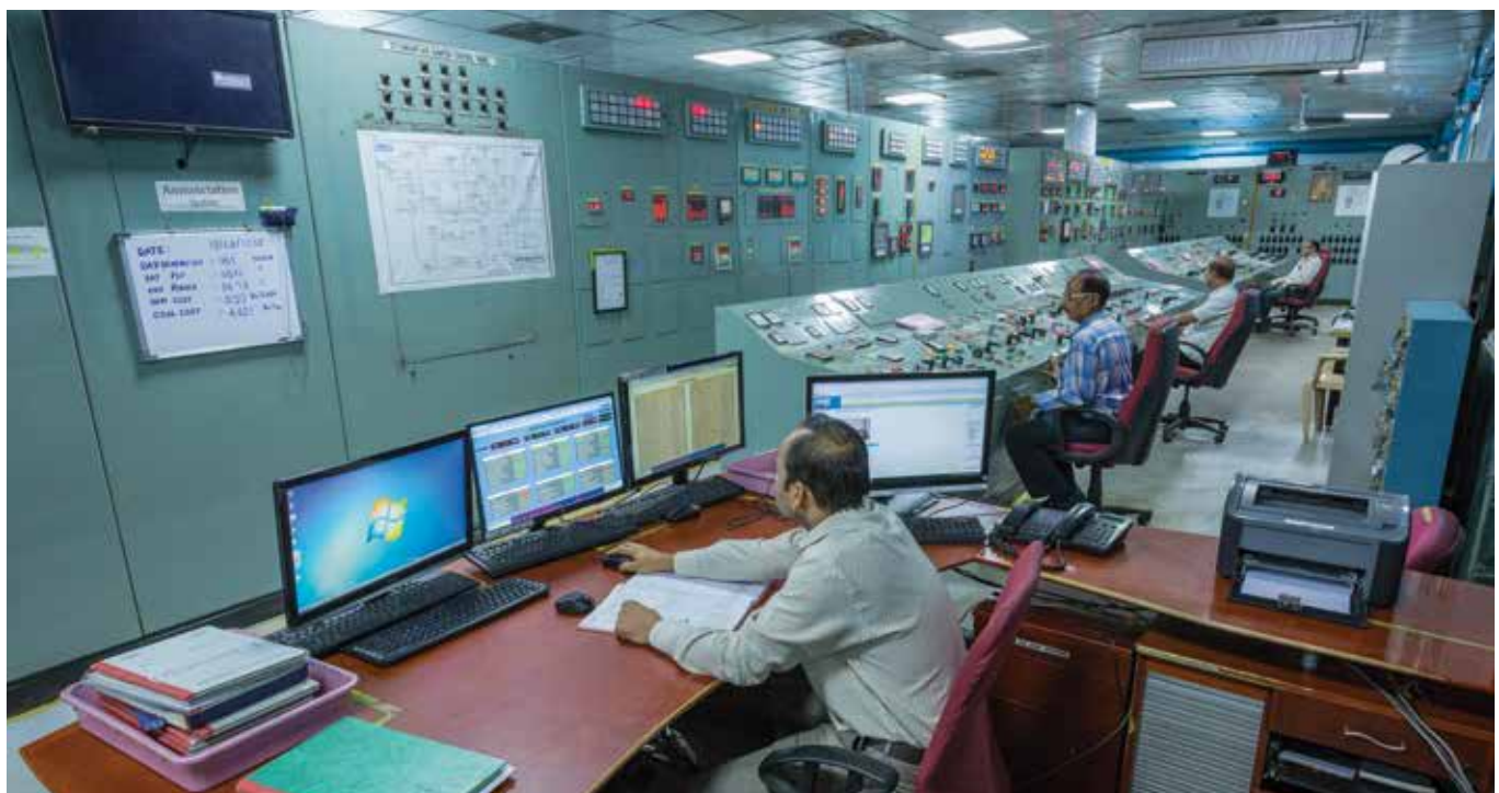
Control Room Bhilai Expansion Project
