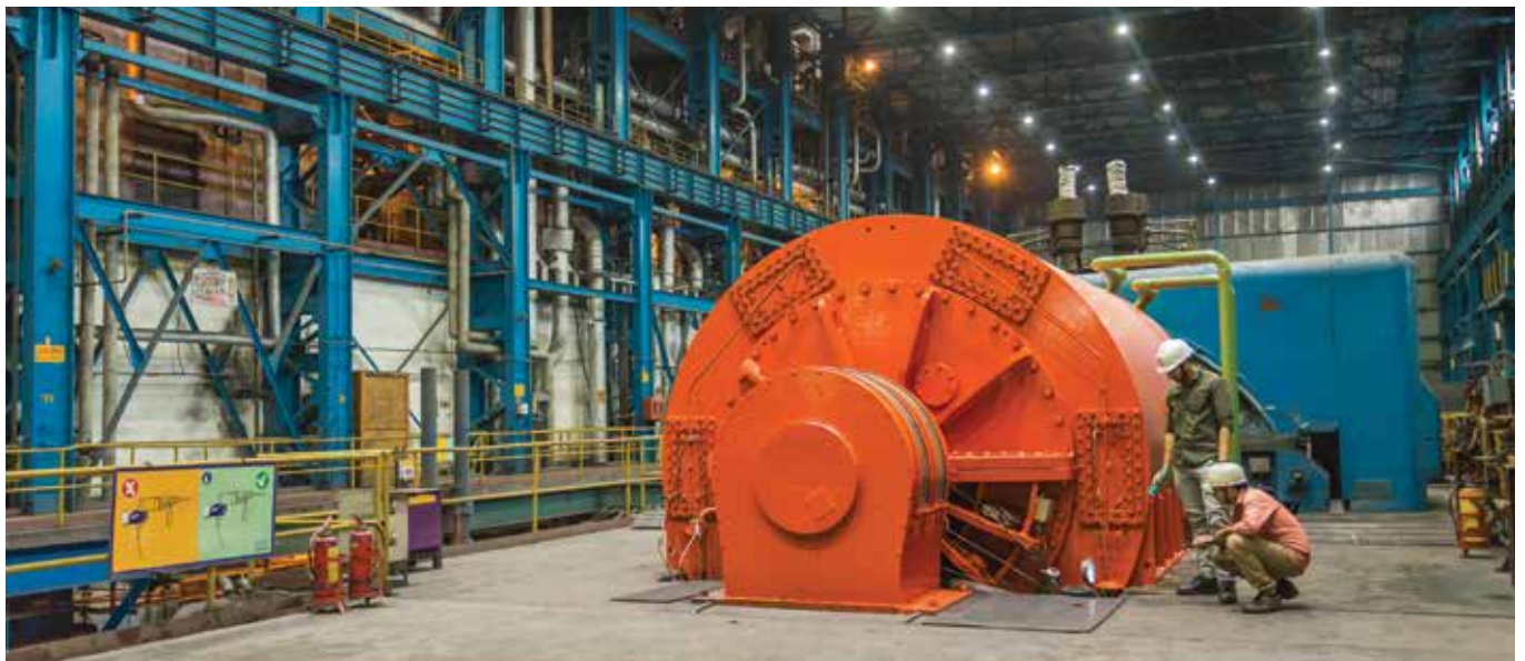
TG Floor NSPCL Durgapur
